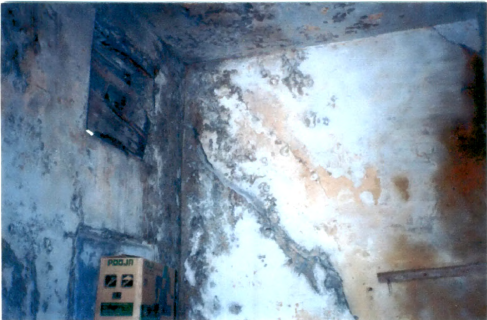
Cracking and flaking off due to dampness in building
