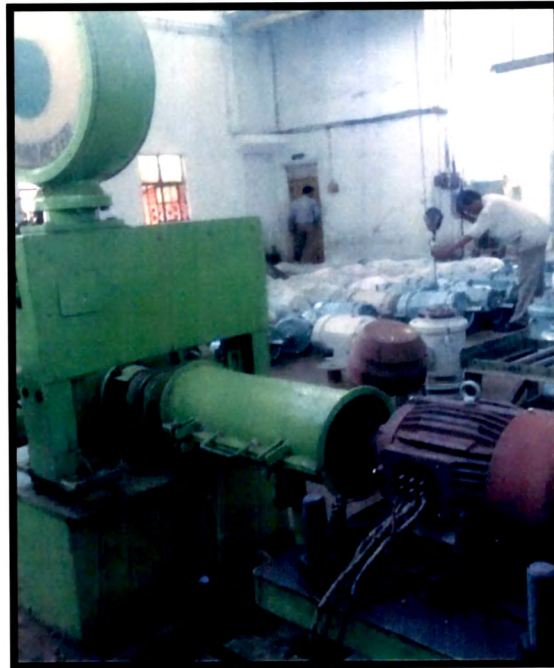
Photograph 3.5. Load test when ABC energized
