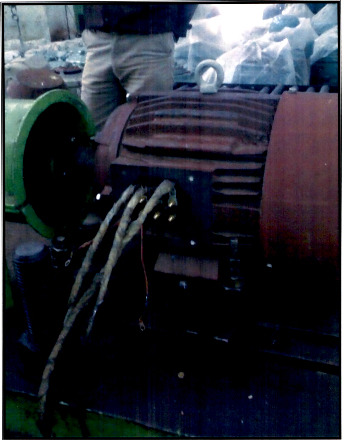
Photograph 3.6. Load test when XYZ energized.
