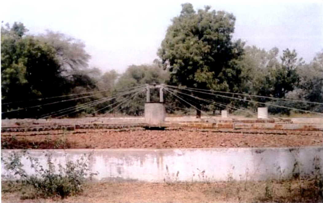
Fig. 4.4 Trickling Filter at Sewage Treatment Plant, Jaspur, Gandhinagar
