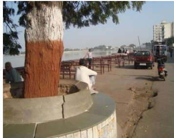
Broken road in Bhuj
