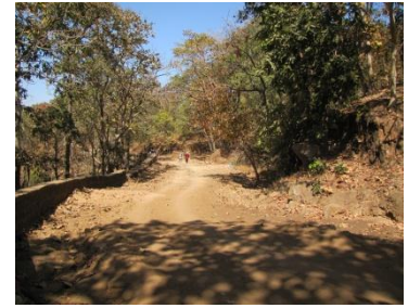
Road Condition at Ratanmahal
